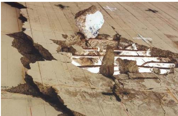
Punching shear (two-way shear) failure
