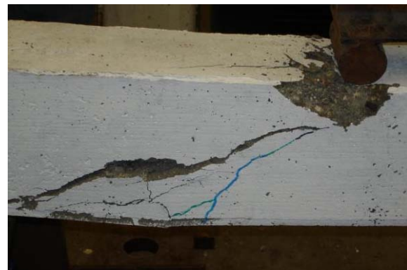
Beam shear (one-way shear) failure
